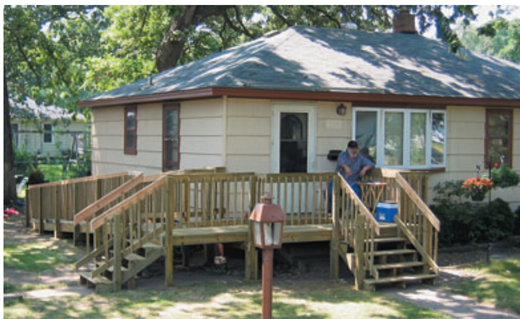
This modular ramp was built over a weekend by Boy Scout volunteers. The Minnesota Ramp Project has the facts.
